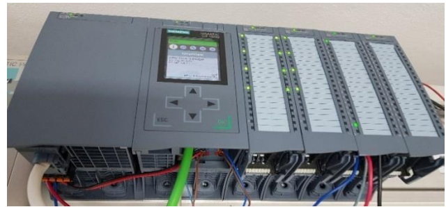
Figure 3. The used PLC control system for data processing The real-time pulses (4 ms) are generated by PLC for measuring with a laser sensor as it is shown in Fig. 4.
