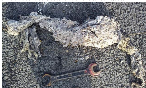
Figure 5. The material of the pressure sewer pipelines, which got clogged due to the influence of combination of underpressure and the lack of flushing speed
