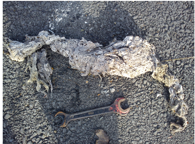
Figure 3. Solids from the wastewater form the clogging in the pipeline of the low pressure sewer network and is gradually completely blocked
