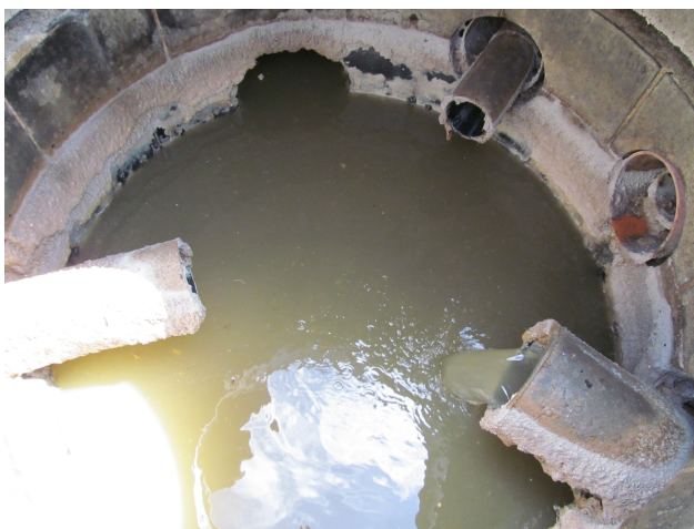
Figure 2. The detail of the outfalling of two separate systems of low pressure sewer network into a common manhole of the gravity sewer network in the wastewater treatment plant
