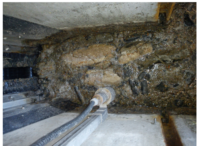
Figure 4. After the unblocking of the clogged pipeline the flushing of the segment is done by a pressure truck; rakings formed into the shape of long cylinders are flushed from the pipeline into the wastewater treatment plant, photo inflow to the wastewater treatment plant
