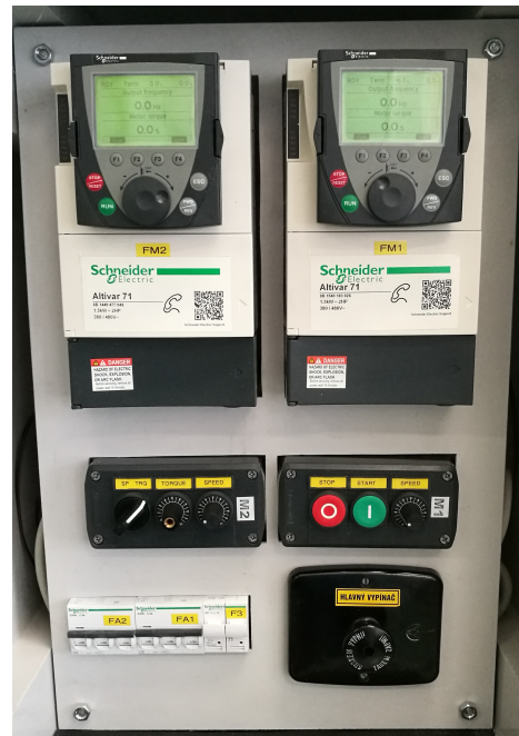
Figure 5. Control panel with frequency converters
