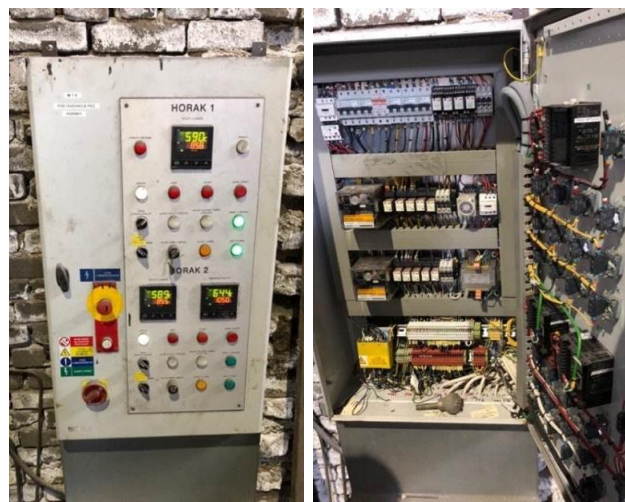
Figure 3. The electro-switch device for controlling performance of burners in the gas melting furnace KOV 010/1998
