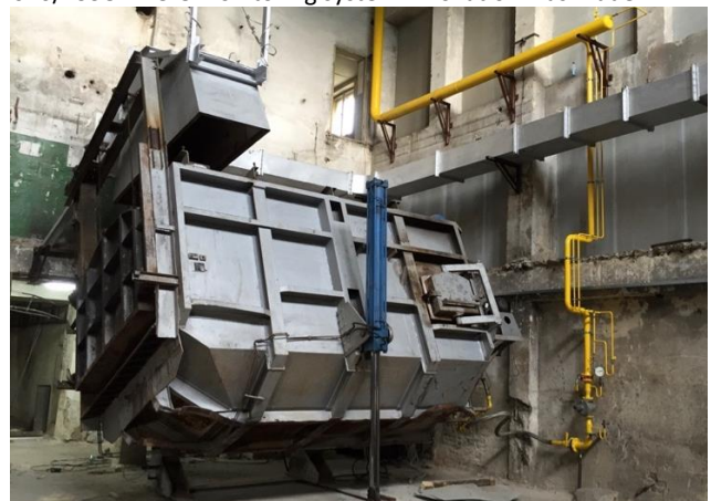
Figure 1. Gas melting furnace KOV 010/1998
