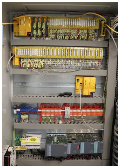
Figure 1. One of the safety control distribution cabinets
