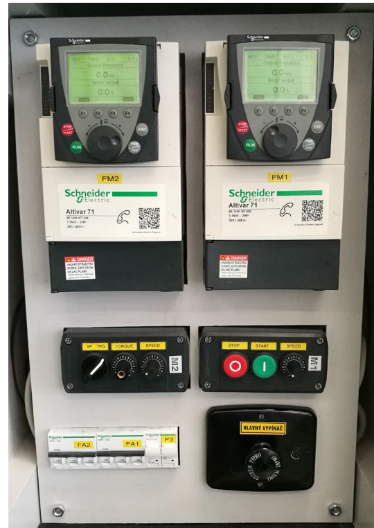
Figure 9. Control panel with frequency converters
