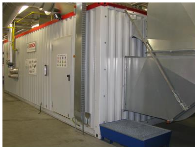
Figure 2. Container with cogeneration unit included inside
