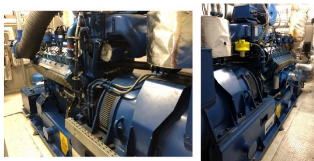
Figure 1. Cogeneration unit engine with generator
