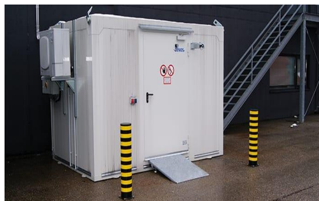
Figure 1. Warehouse of Li-ion accumulators
