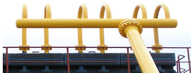
Figure 2. One section of the cooler – 3 blocks
