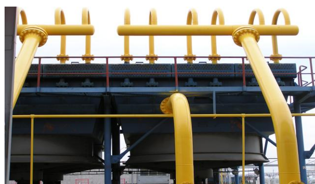
Figure 1. Natural gas cooler – a detailed image of the fan section
