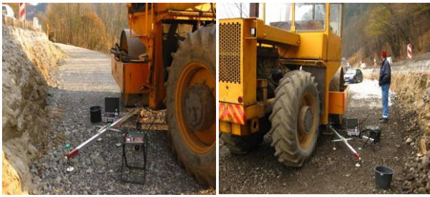
Figure 3. Application of Simat 32/64 mm in rehabilitation of landslide road (archive Viliam Hires)
