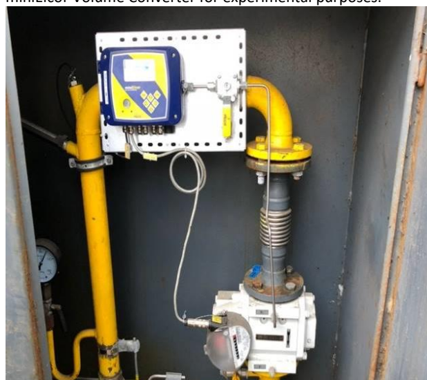
Figure 3: Digital gas meter ELGAS miniElcor Volume Converter
