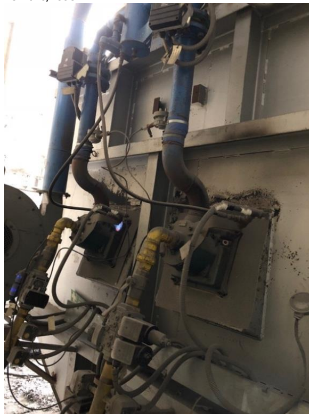
Figure 2: The system of burner no. 1 and no. 2 including the air supply to the melting furnace KOV 010/1998
