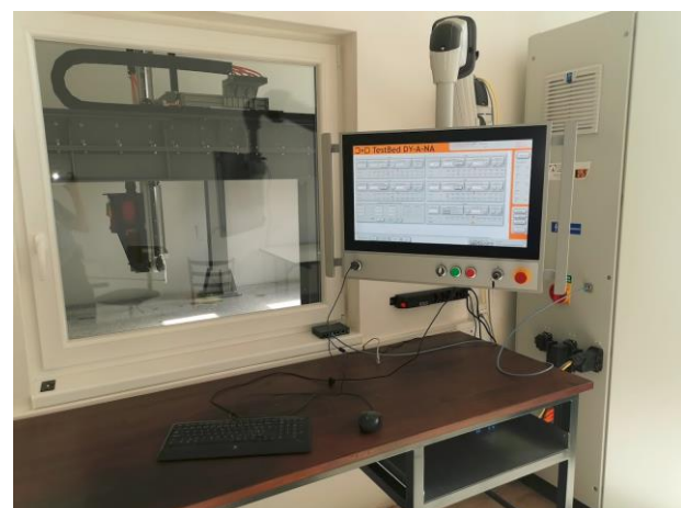
Figure 9. Control panel with HMI
