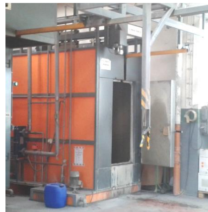
Figure 11. Pre-surface treatment cabin
