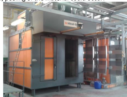
Figure 5. Hot air furnace
