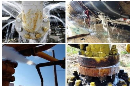
Figure 1. Different types of damage to the pipeline and its components [SEPS 2022]
