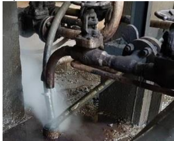
Figure 21. Closure leak DN50 [SEPS 2022]
