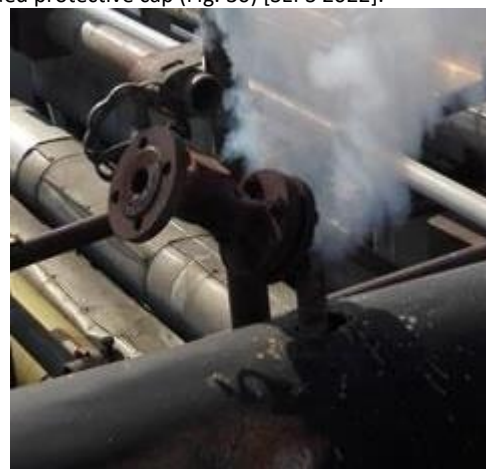
Figure 26. Torn off closure of the steam line in the weld under the flange [SEPS 2022]
