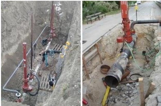
Figure 18. Use of bypass in case of a need of continuous supply of product in a pipeline [SEPS 2022]
