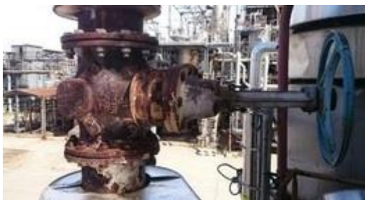
Figure 23. Torn off spindle of the closure plate in a closed position [SEPS 2022]
