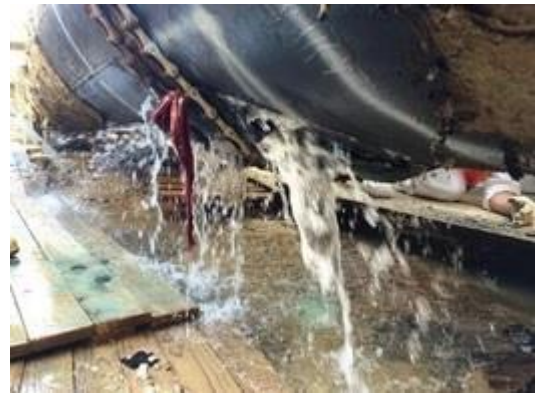
Figure 3. An unsuccessful attempt to stop the water leak by patch [SEPS 2022]
