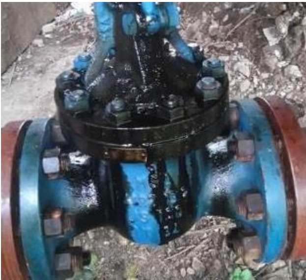
Figure 13. Leak outside the closure [SEPS 2022]
