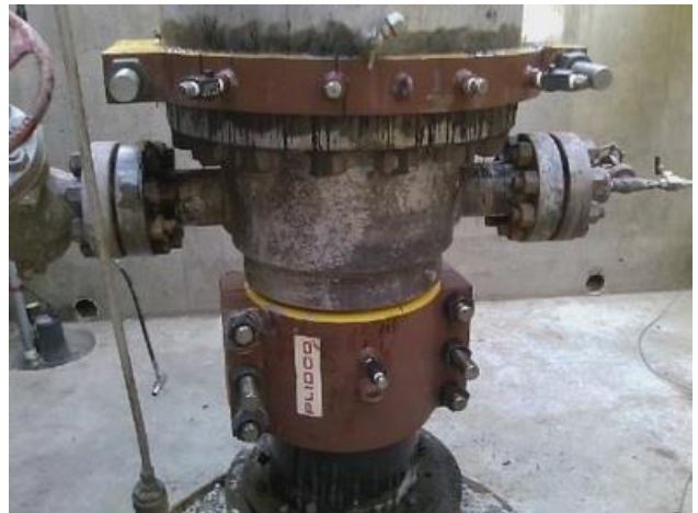
Figure 10. Flange joint leak stop [SEPS 2022]
