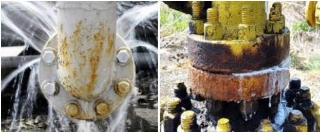
Figure 7. Leaks at flange joints [SEPS 2022]
