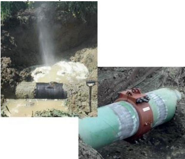
Figure 2. Pipe leak and split sleeve PLIDCO Split+Sleeve [SEPS 2022]
