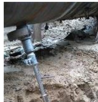
Figure 4. Insertion of the plug after the installation of a sleeve with a leak diversion [SEPS 2022]
