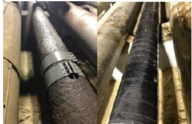
Figure 5. Stopping of the leak using a steel strap with a rubber seal [SEPS 2022]
