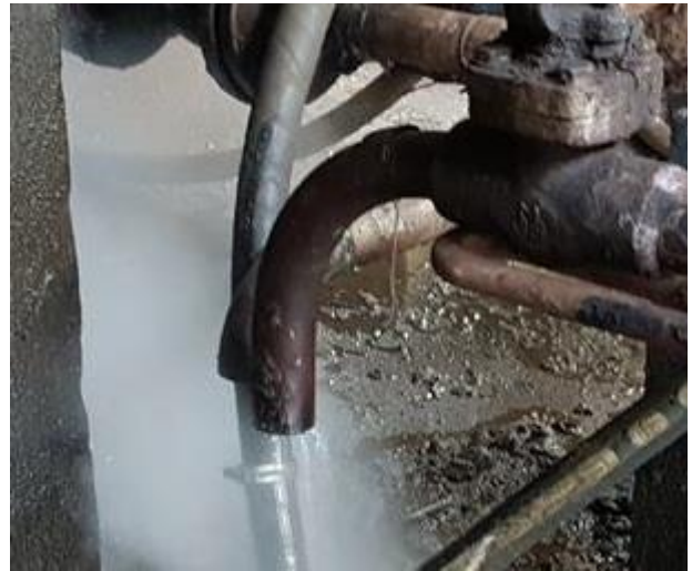
Figure 14. Leak through the closure [SEPS 2022]
