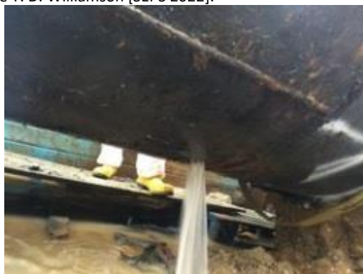
Figure 2. Water leak through a hole in a pipe [SEPS 2022]
