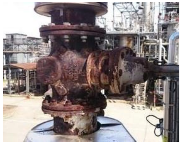
Figure 15. Torn off plate of the closure [SEPS 2022]
