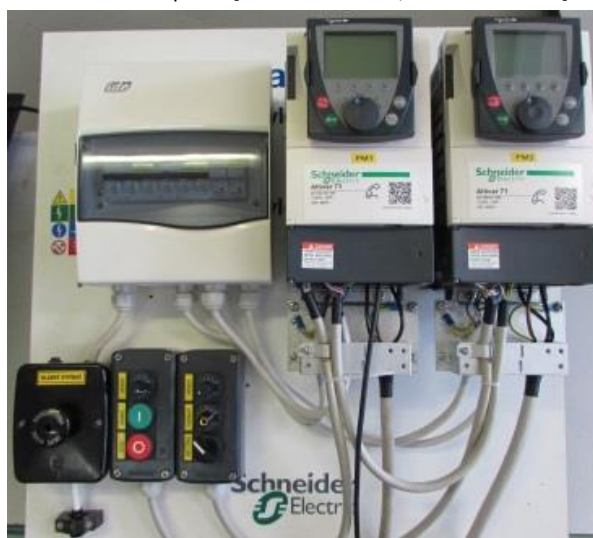
Figure 1. Control panel of testing device
